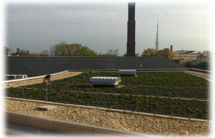
Roof Space with Native Landscaping at Woodrow Wilson High School
