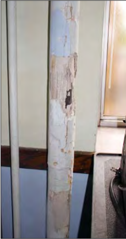
Deteriorating pipes can put students and staff in danger of falling debris and unknown contaminants.
