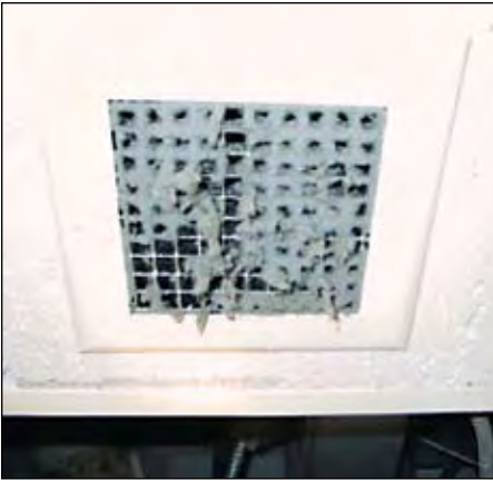
Many problems are maintenance issues, such as this long-neglected air vent.
