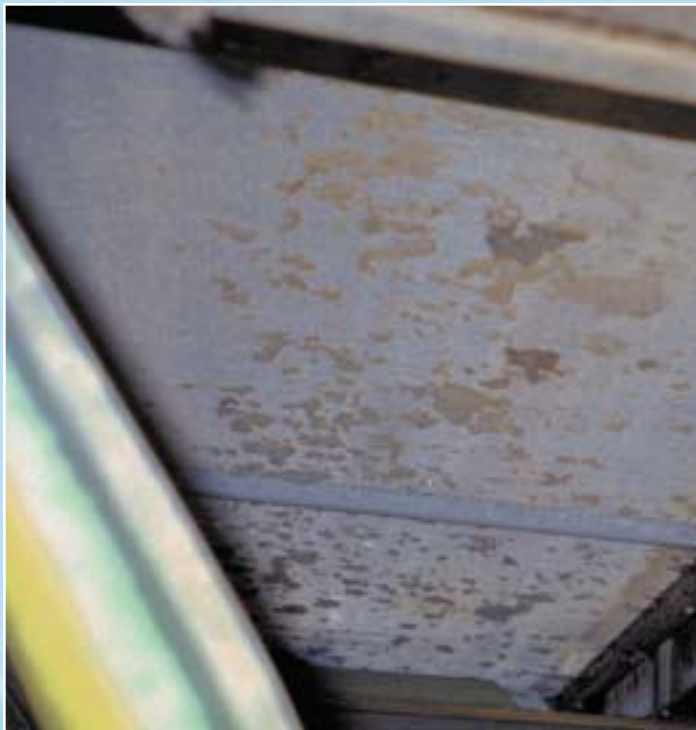
Mold on ceiling in a Georgia elementary school, photo by Daniel Friedman
