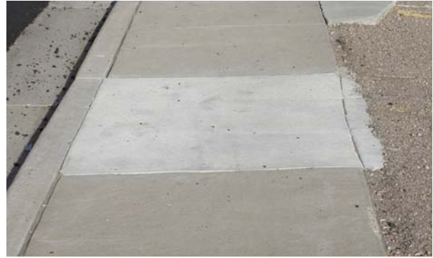
Sidewalk sections should be replaced where tree roots or other problems have created irregular surfaces.
