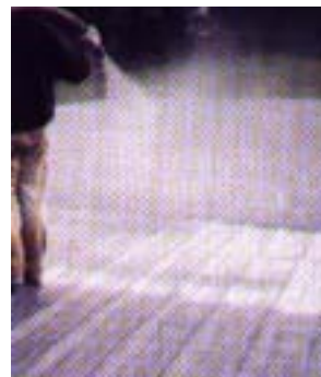
Elastomeric or other coating can be field applied to many roof substrates.
