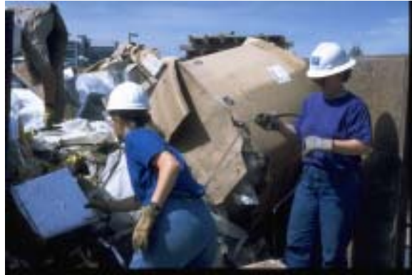
A construction site waste audit can help reduce waste generated and divert materials through processes from disposal through reuse and recycling. NREL/PIX 11407
