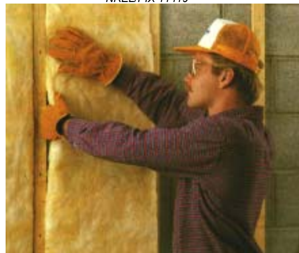
Masonry walls can be insulated on the interior, but the benefits of thermal mass are mostly lost.
