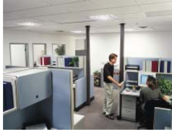
Tubular skylights in interior administrative office provide high lighting levels even when electric lights are off. Skylight diffuser panel fits into a standard suspended ceiling system.
