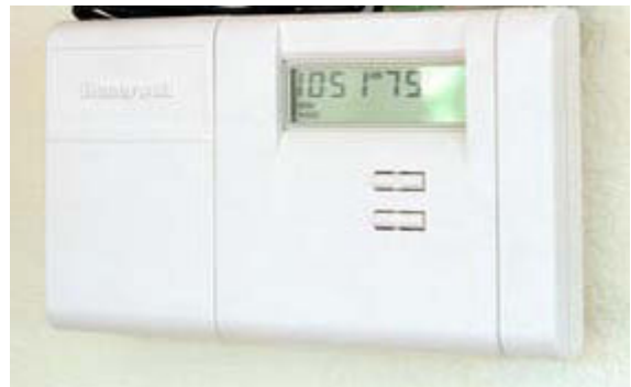
Adjustable thermostats allow the user to have control over the conditions of the room, which can improve overall comfort and create a better learning environment.
